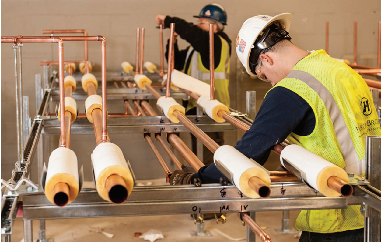
Figure 12. Prefabrication of plumbing racks at Consigli’s Prefab Lab. Source: (Teichloyz, Sarma et al. 2017).
