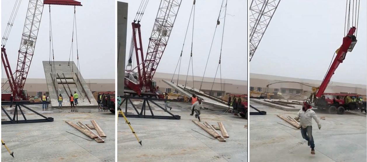
Figure 2. What could go wrong: sequence of a construction accident in Austin TX, involving a precast wall component. Retrieved from: https://youtu.be/Mn6PYOG6sWw .
