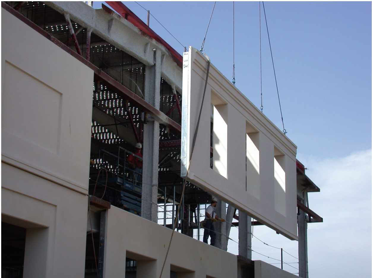
Figure 32. Precast wall panel being hoisted in place. Source: National Precast Concrete Association (NPCA). Retrieved from: http://precast.org/wp-content/uploads/2014/08/Precast-Concrete-Wall-Panel-Install.jpg .
